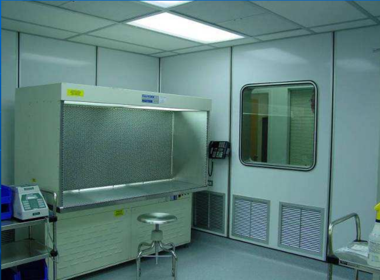
Cleanroom housing primary engineering controls
